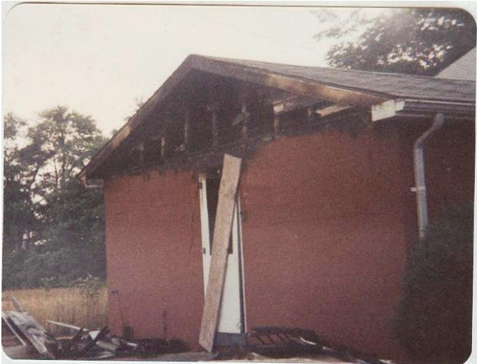
Grange Hall after the June 1988 Fire
